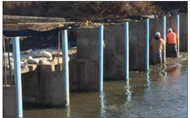
While the emergency work of reinforcing the structure of Sack Dam was being completed, the height of the Dam was raised several feet.
