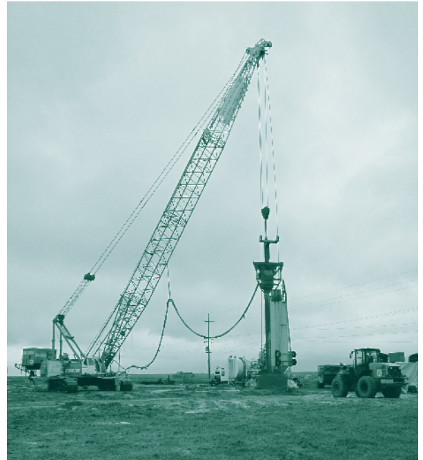
The foundation has been laid on a demonstration drainage water treatment plant to address salt accumulation and other drainage issues in the San Luis Unit. These projects are incorporated in the Exchange Contractors' newly approved Strategic Plan.
